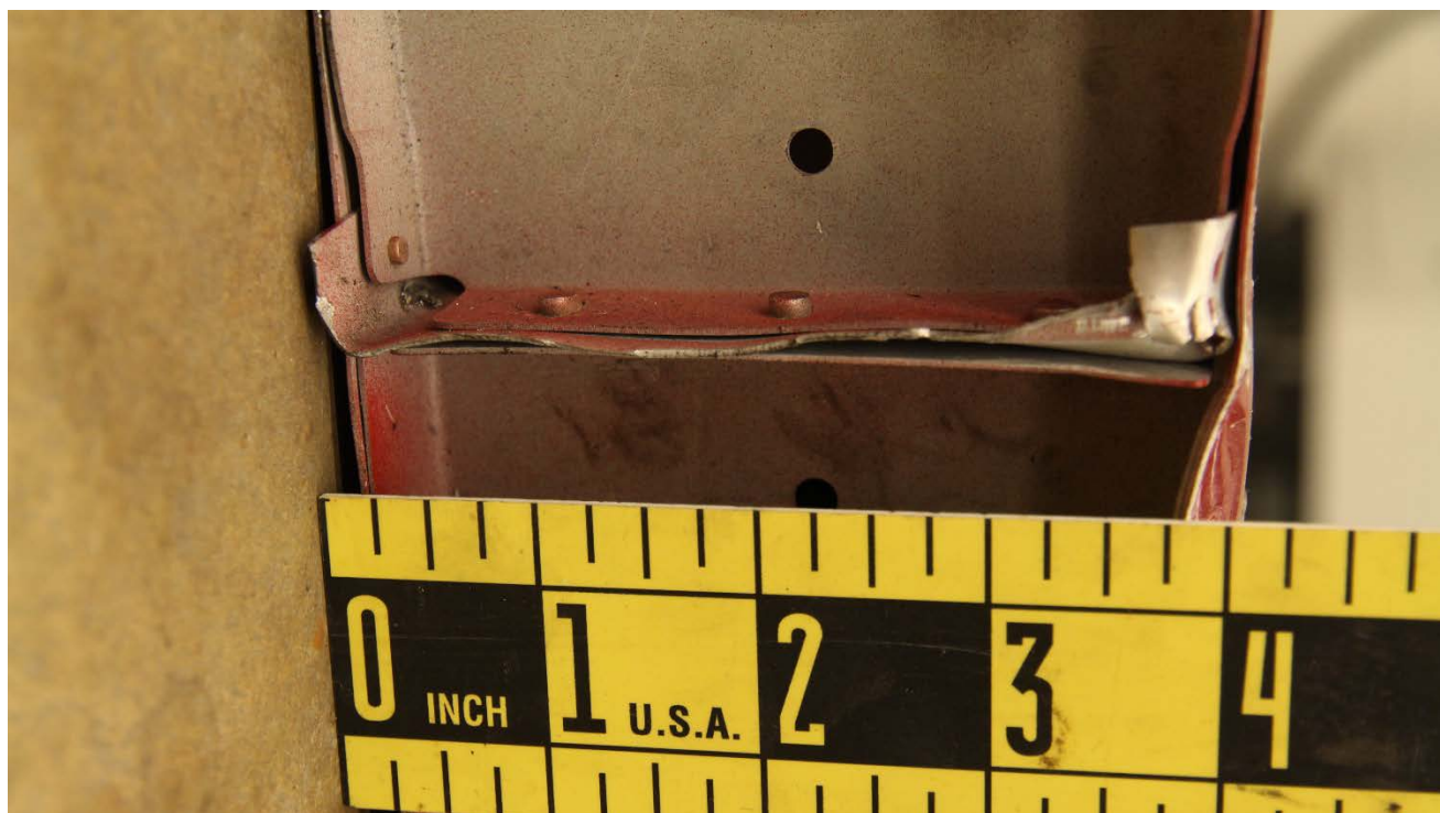
Figure 15 – Closer view of the fracture surface from the forward vertical spar from Figure 14.
