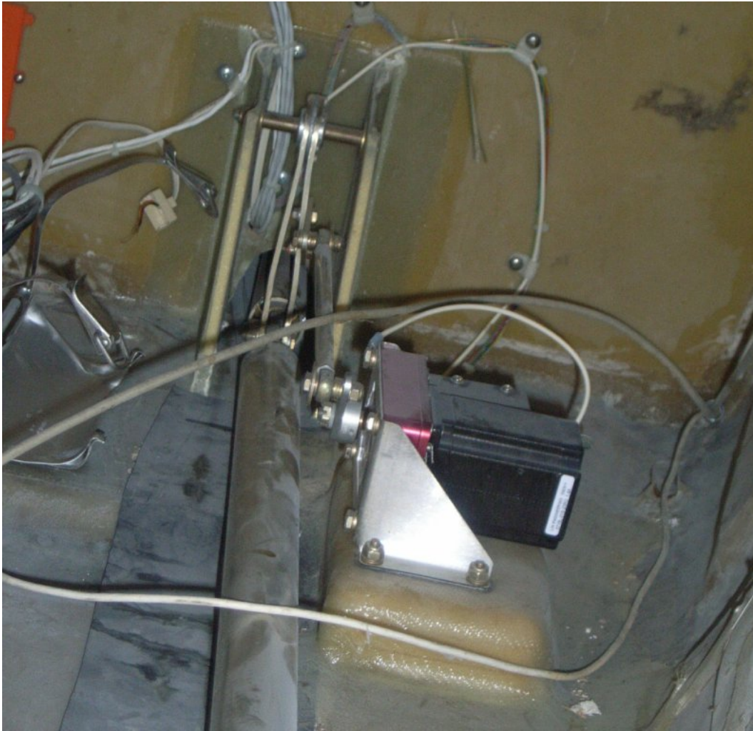
Figure 18 - Elevator Control Rod and Autopilot Pitch Servo
