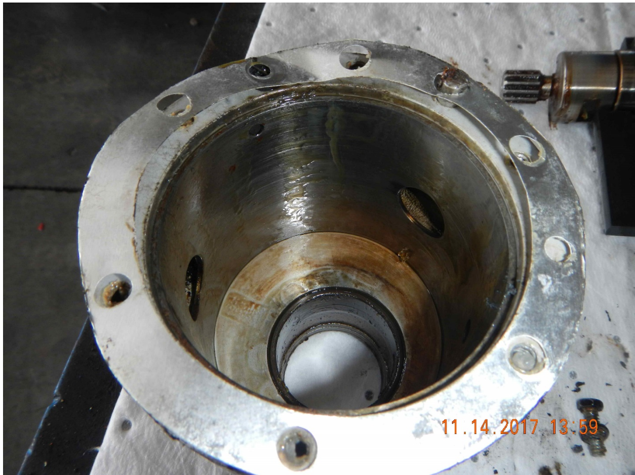
Photo 14 – Vacuum Pump Housing
