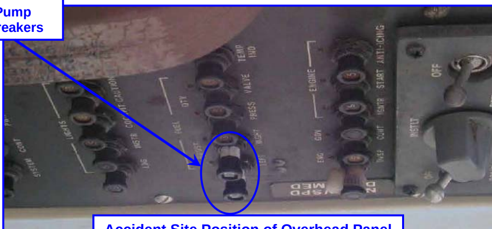
Accident Site Position of Overhead Panel Circuit Breakers
