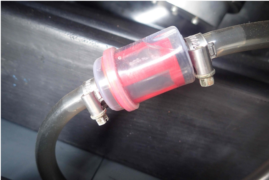
Photo 4 - Fuel Filter and Line after Engine Start
