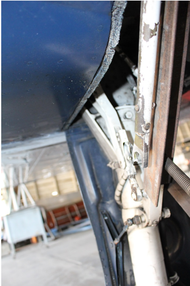
Photograph 2: Right Main Landing Gear Aft Tube Rod End
