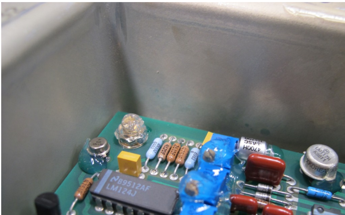
Figure 9 - Control Box Interior Behind Bubbled Paint
