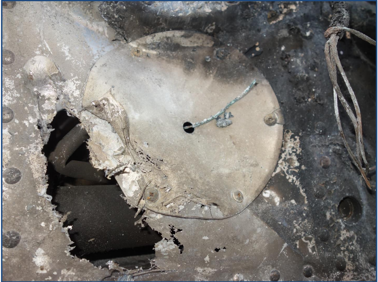
Figure 2: Wire coming through a hole drilled in a cabin floor inspection plate, into the cabin.
