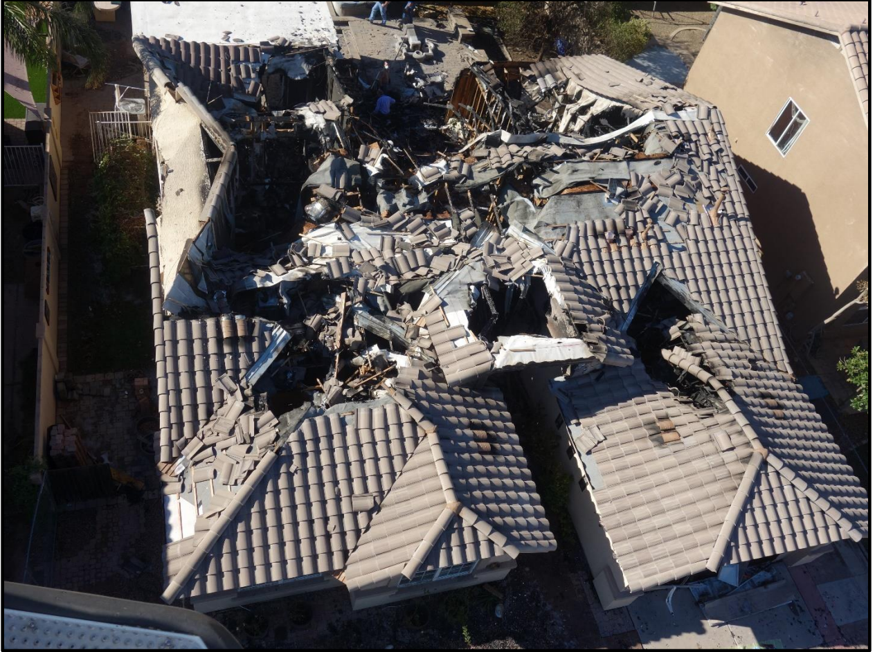
Figure 2: Top view of house damage.
