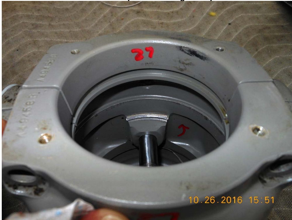
Photo #7 – Left hub L2 blade pocket damage and paint transfer mark
