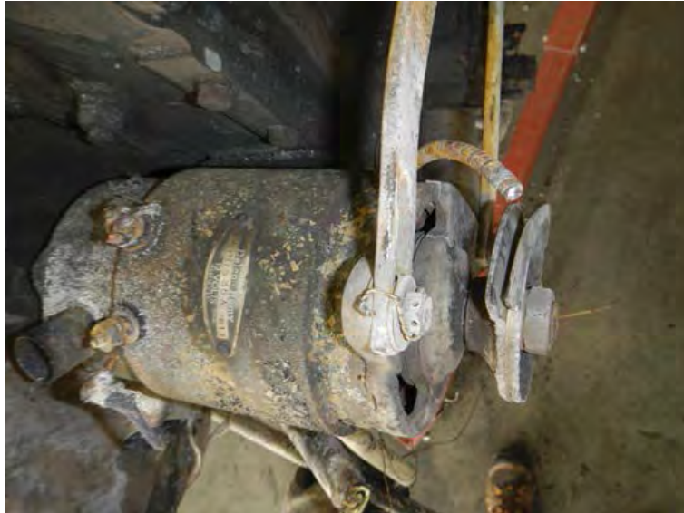
Figure 16 - photo of generator
