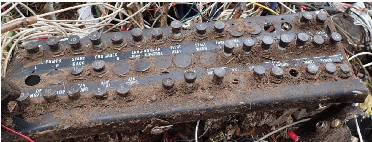
Figure 26 - Circuit Breaker Panel
