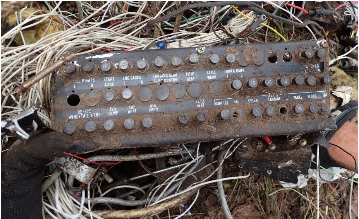
Figure 25 - Circuit Breaker Panel
