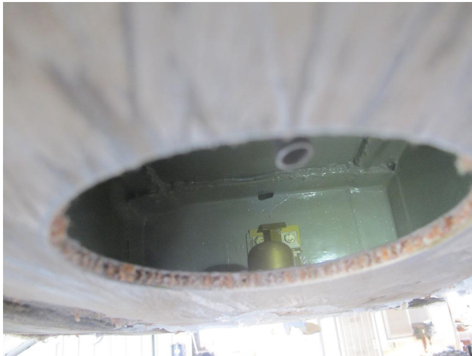
Photo 15 Belly Drain in Front Center Compartment
