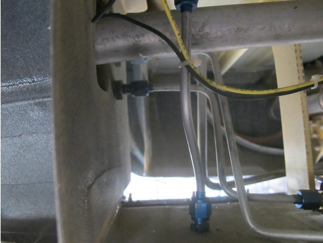
Photo 19 Vent Connection to Belly Tank
