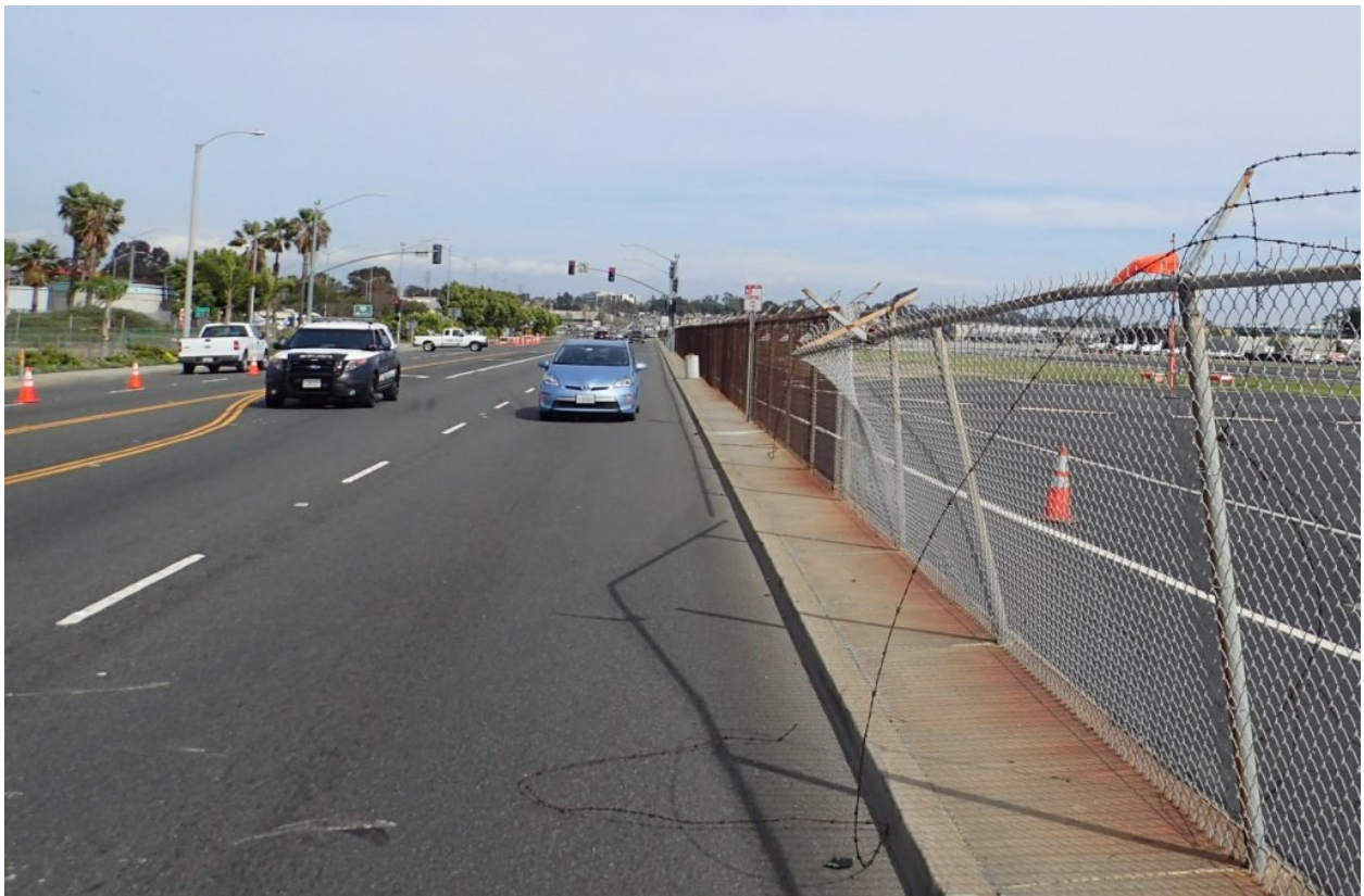
Figure 5 - Fence Damage and Ground Scars (looking east)
