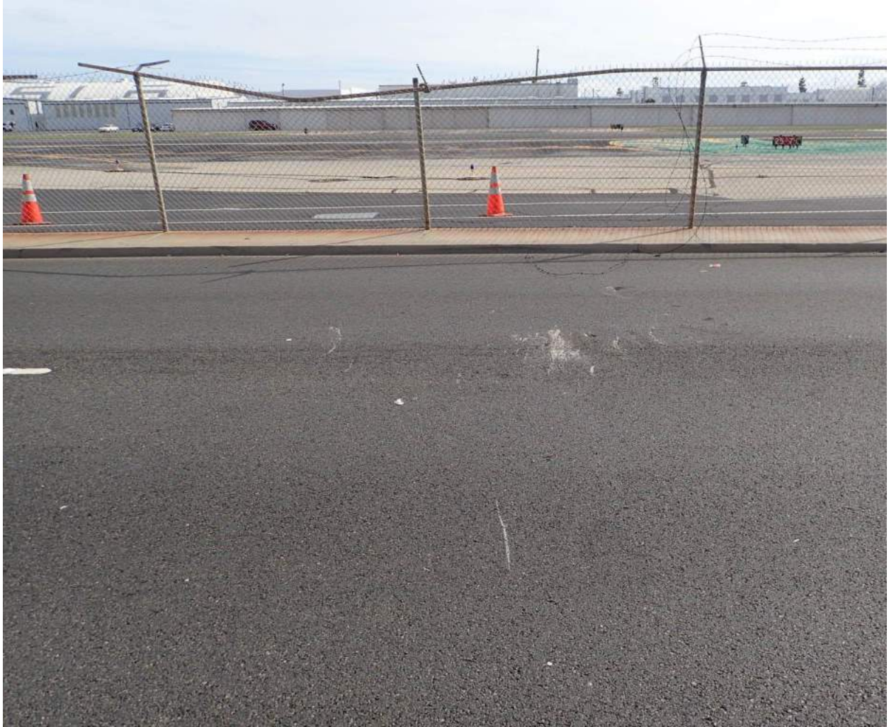
Figure 6 - Fence Damage and Ground Scars (looking south)
