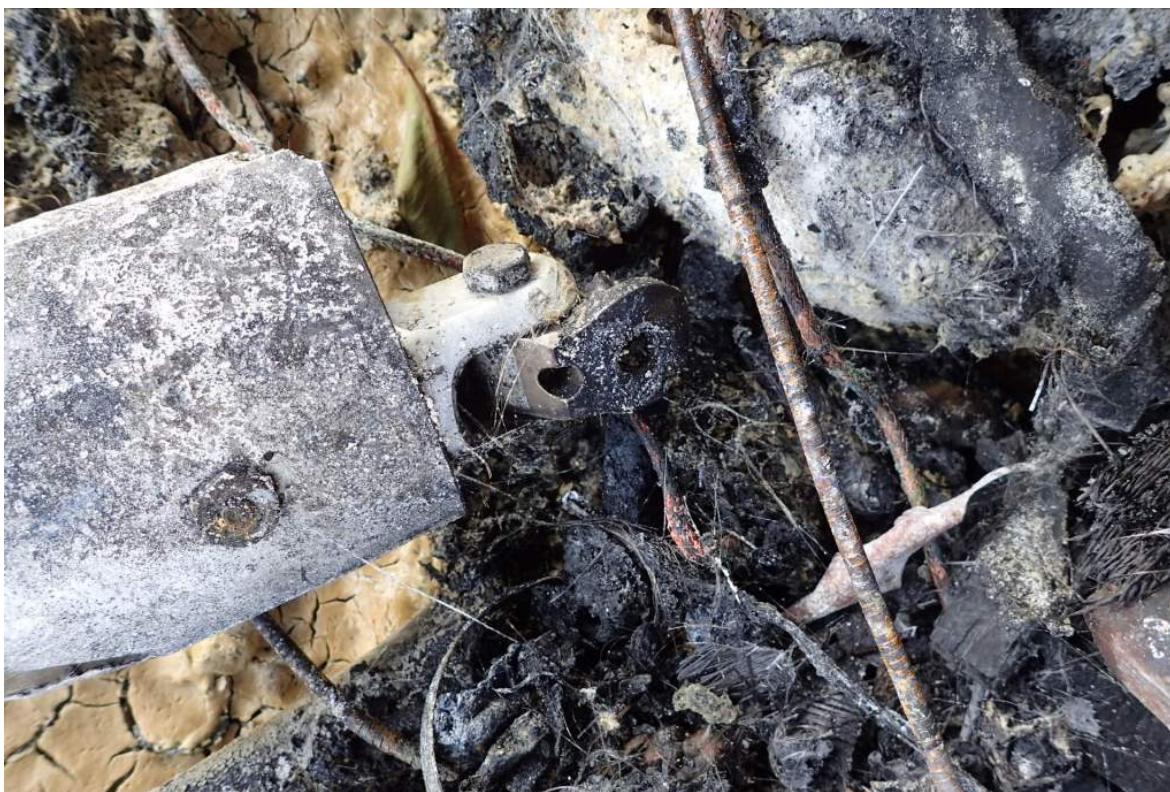
Figure 33 - Fractured Upper Left Strut Attach
