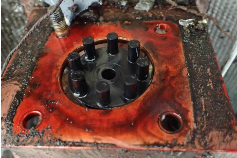
Photo 12 – Secondary Vacuum Pump Drive Pins
