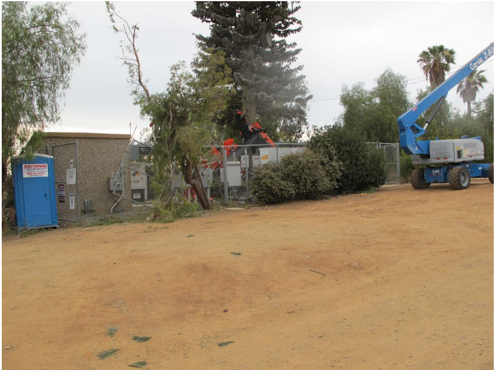
Photo 3 – Looking at Site in Direction of Debris Field
