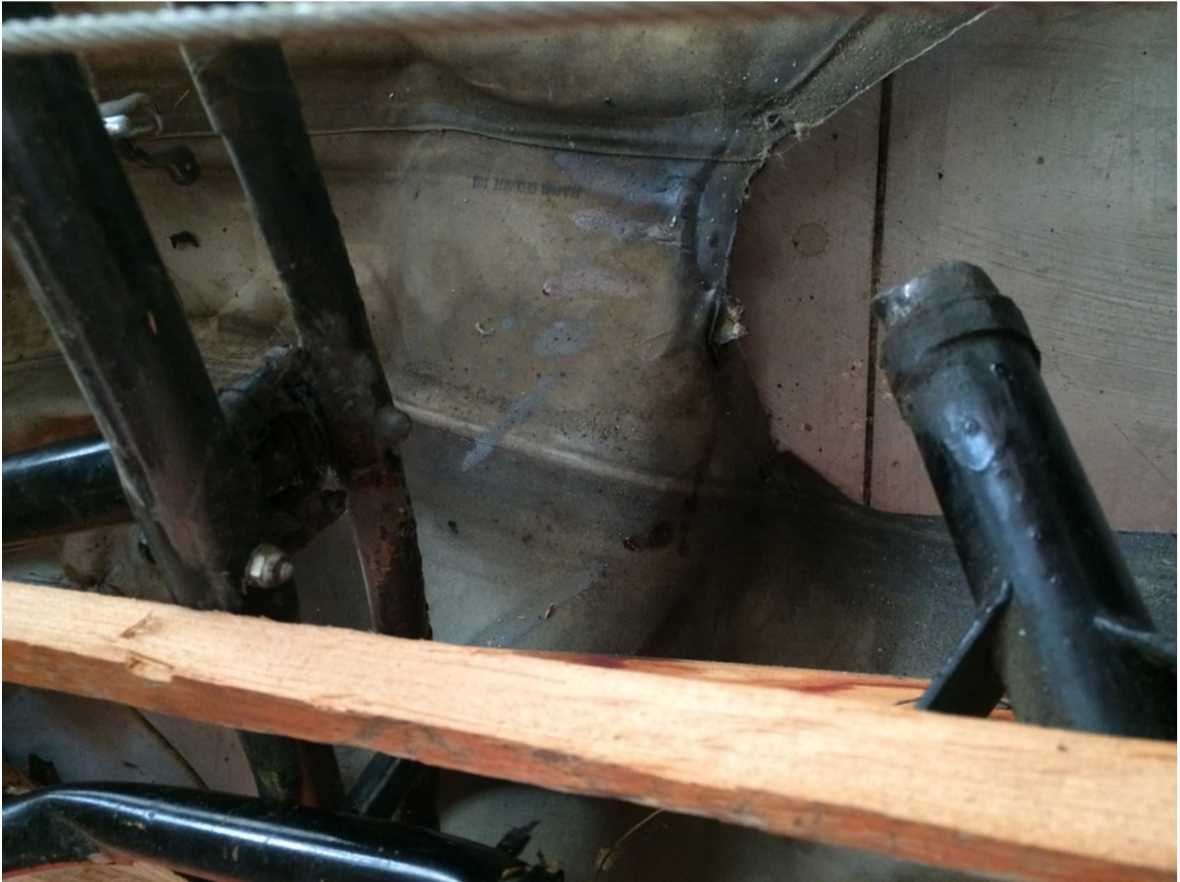
Photo 2 – Close-up of Fractured Tube
