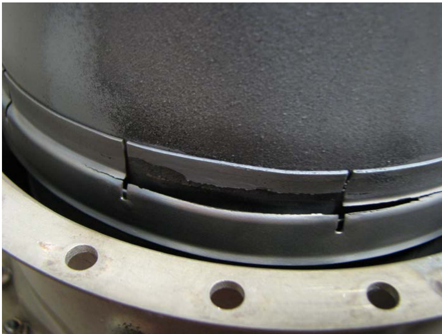
Figure 16 – Combustor Liner – Detail of Crack at Fishmouth Seal
