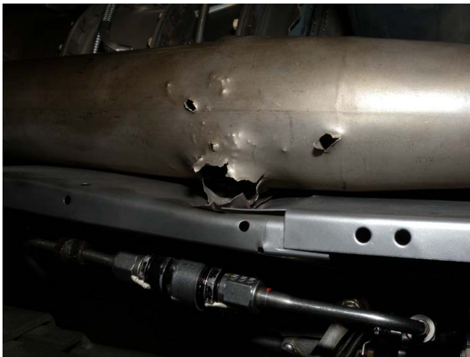
Figure 14 – Detail of Compressor Discharge Tube Damage - Outside
