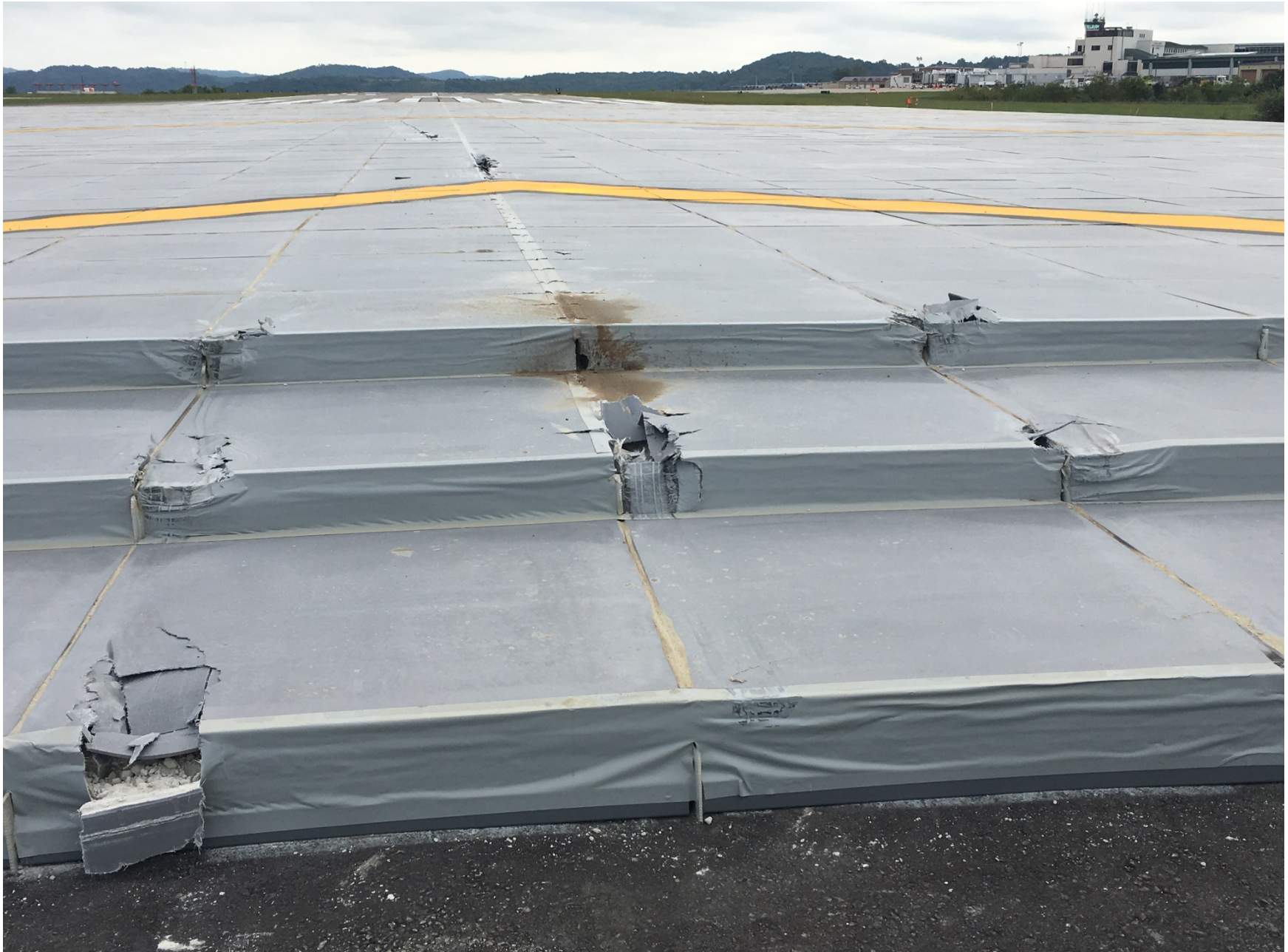
Photo 1 – View of impact markings on engineered material arrestor system (Photo courtesy of the FAA)
