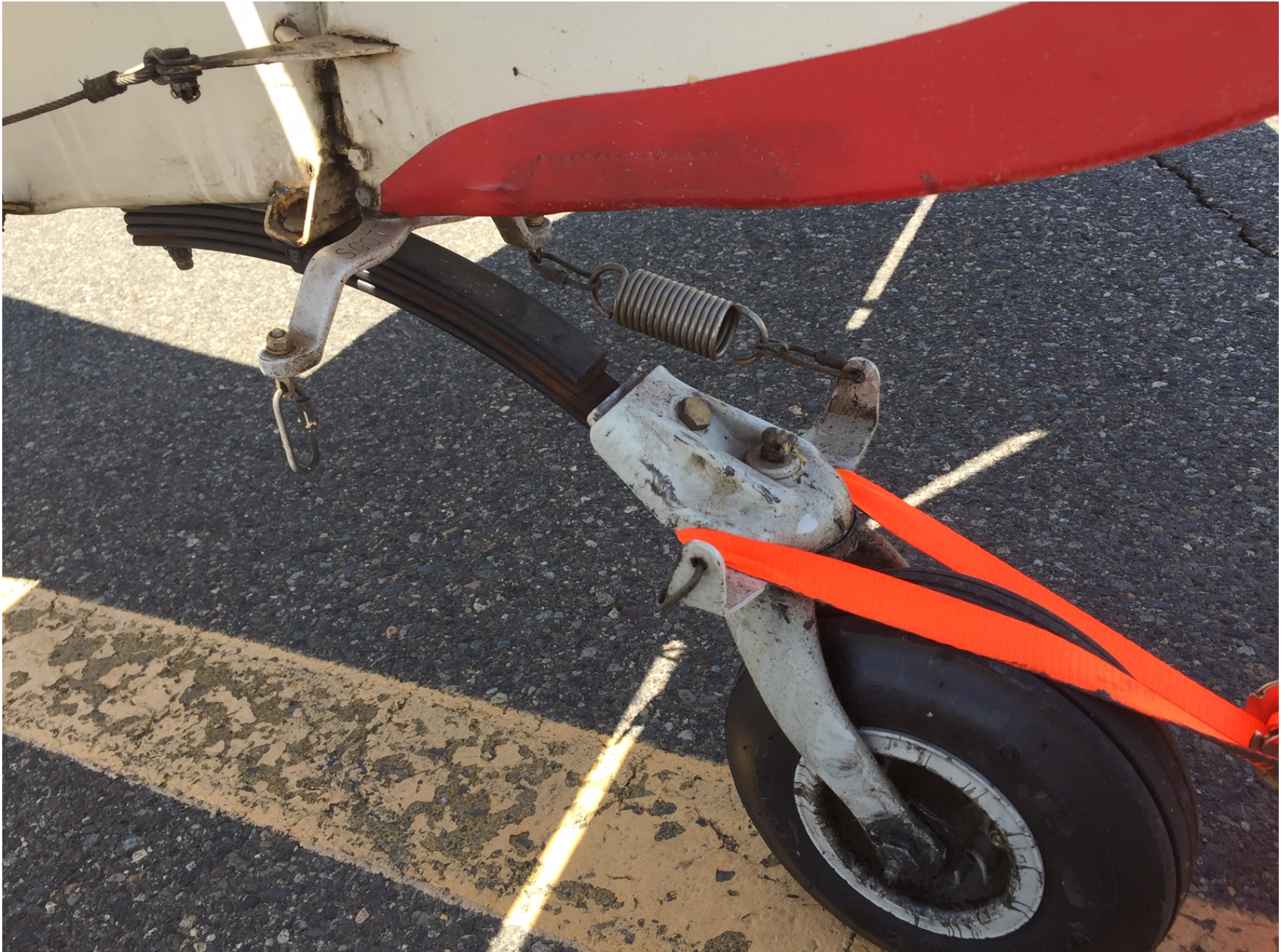
Photo 2 – View of tailwheel assembly with missing left steering spring (Photo courtesy of the airport manager)
