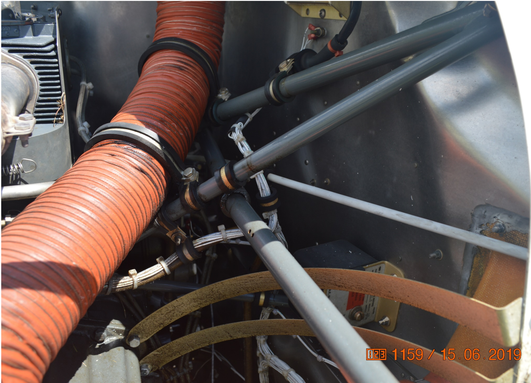
Photo 2 – View of damaged firewall (Photo courtesy of the FAA)
