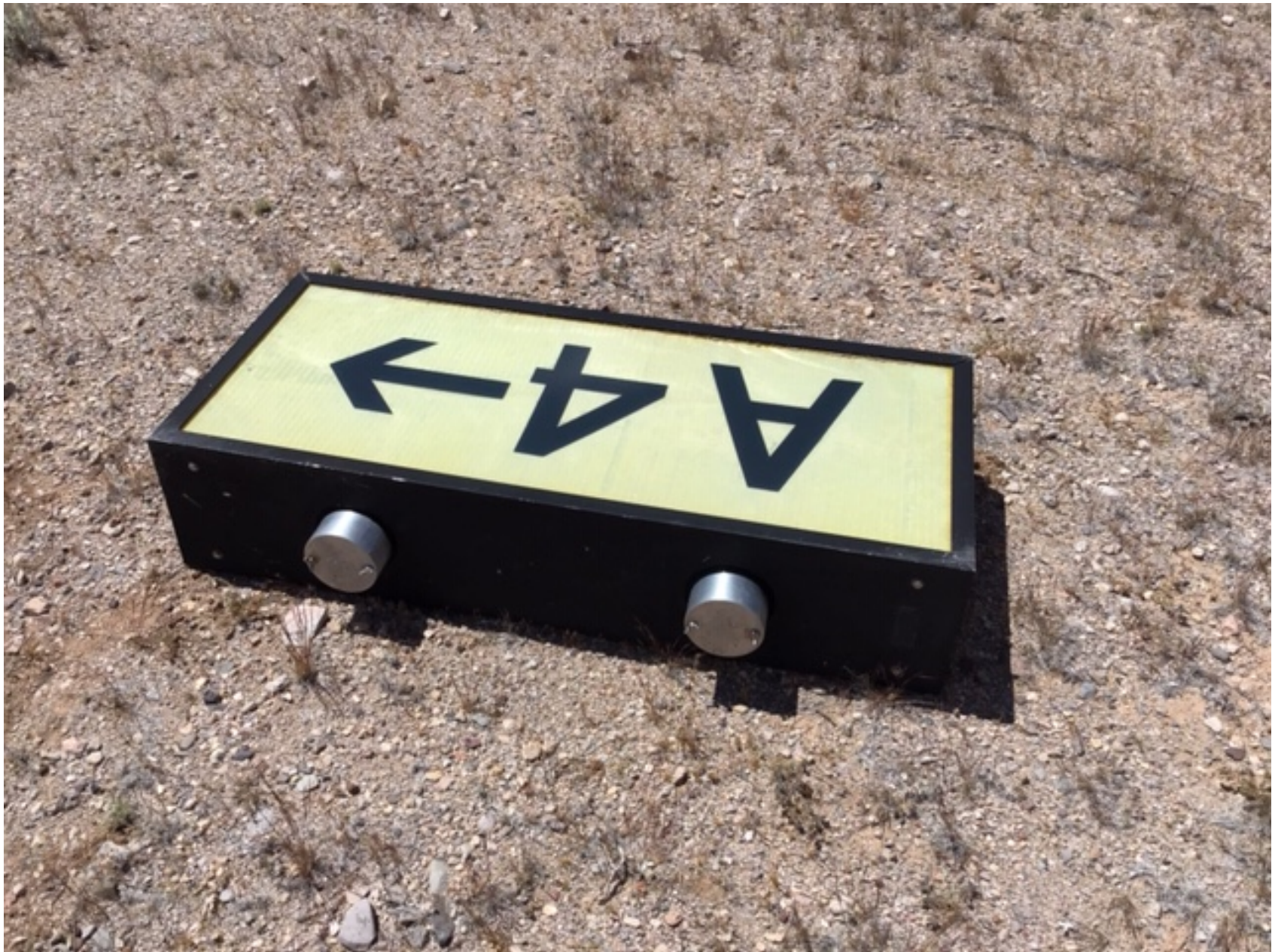
Photo 3 - View of damaged airport taxi way sign (photo courtesy of the FAA)
