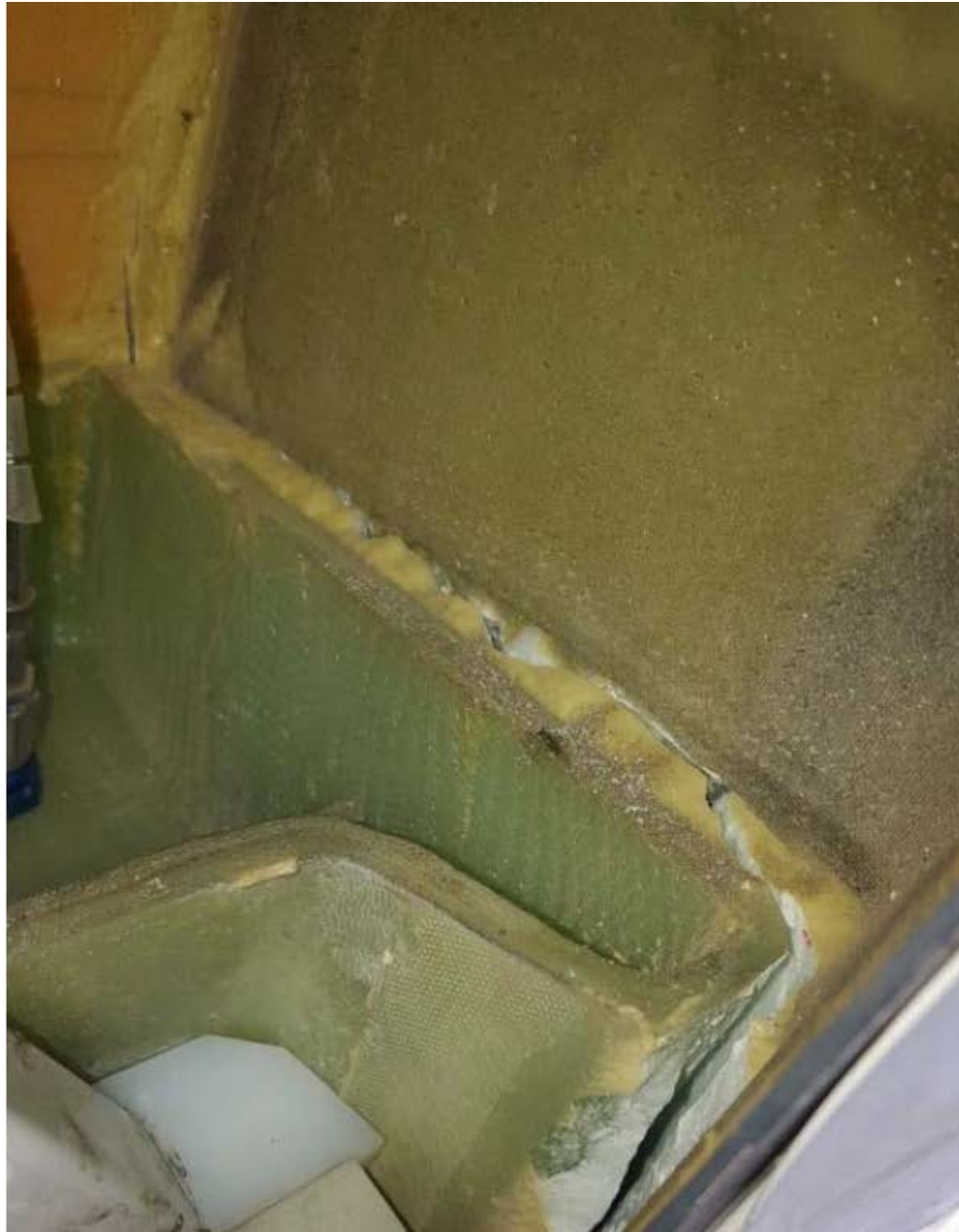
Photo 2 – View of damage to the right main landing gear attachment mount and composite structure -Image was taken with the tail of the airplane to the right (Courtesy of FAA)
