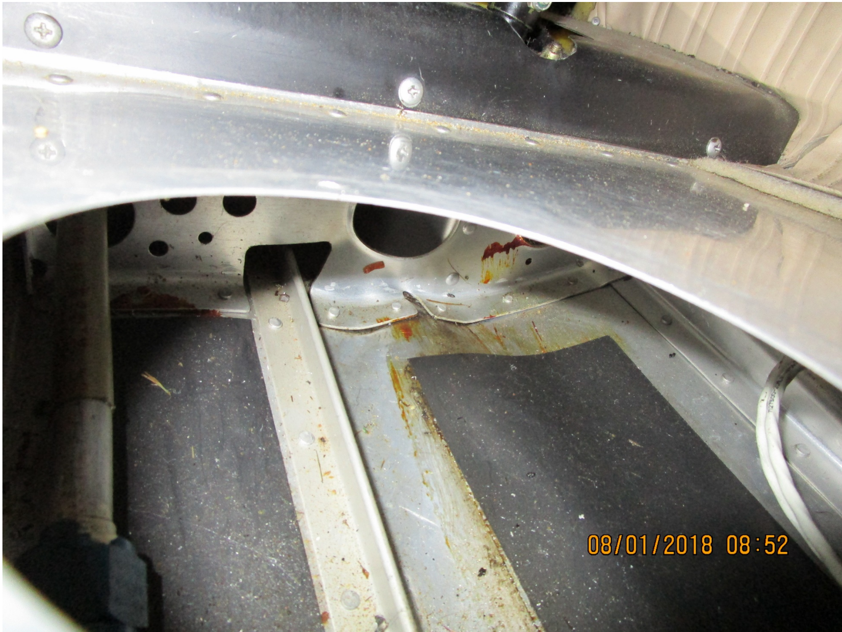
Photo 2 – View of damaged floorboards (Photo courtesy of the FAA)
