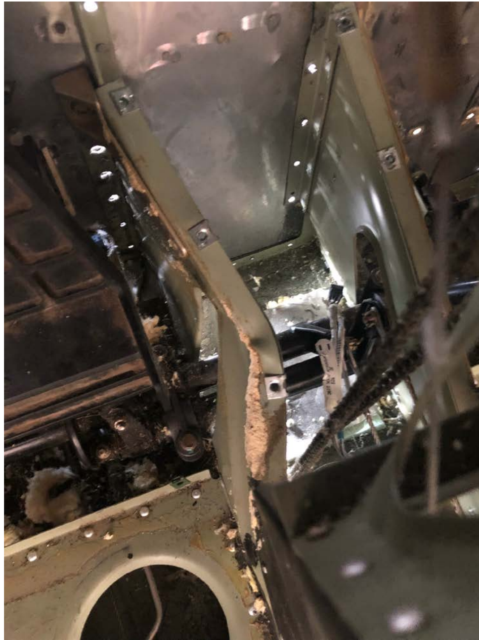
Photo 1 – View of damage to left side tunnel for the nose landing gear (courtesy of the FAA)
