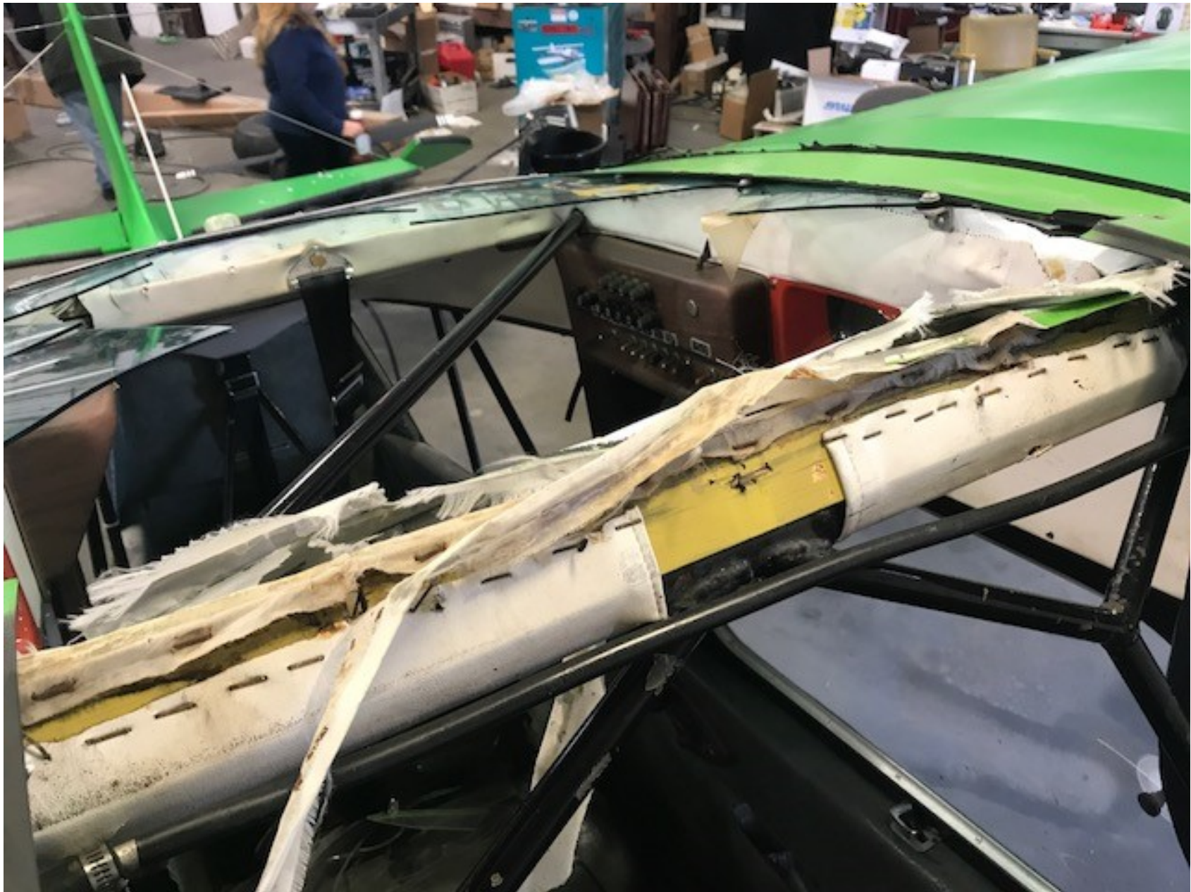
Photo 2 – View of retainer windshield top missing through-bolts and greenhouse support (Courtesy of FAA)
