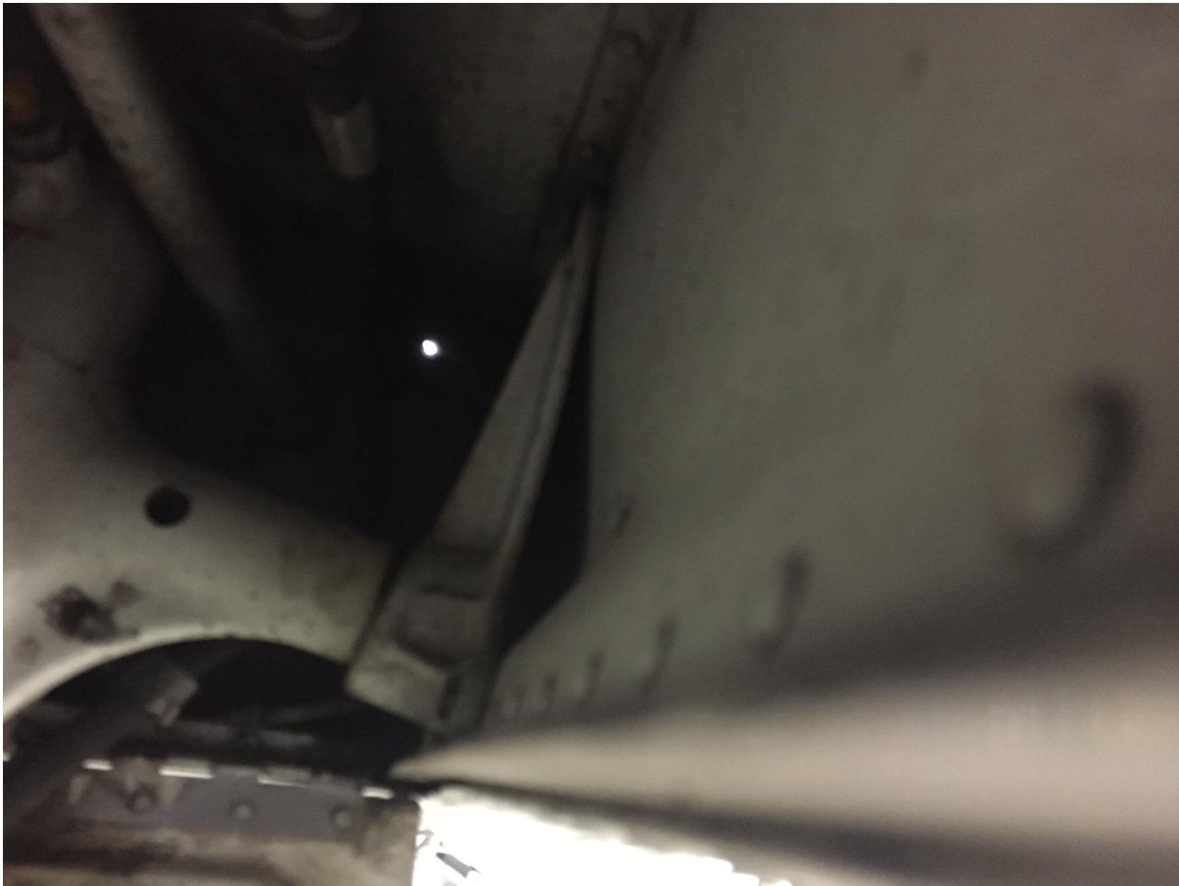
Photo 1 – View of right wing spar damage looking up from right landing gear well (photo courtesy of FAA)
