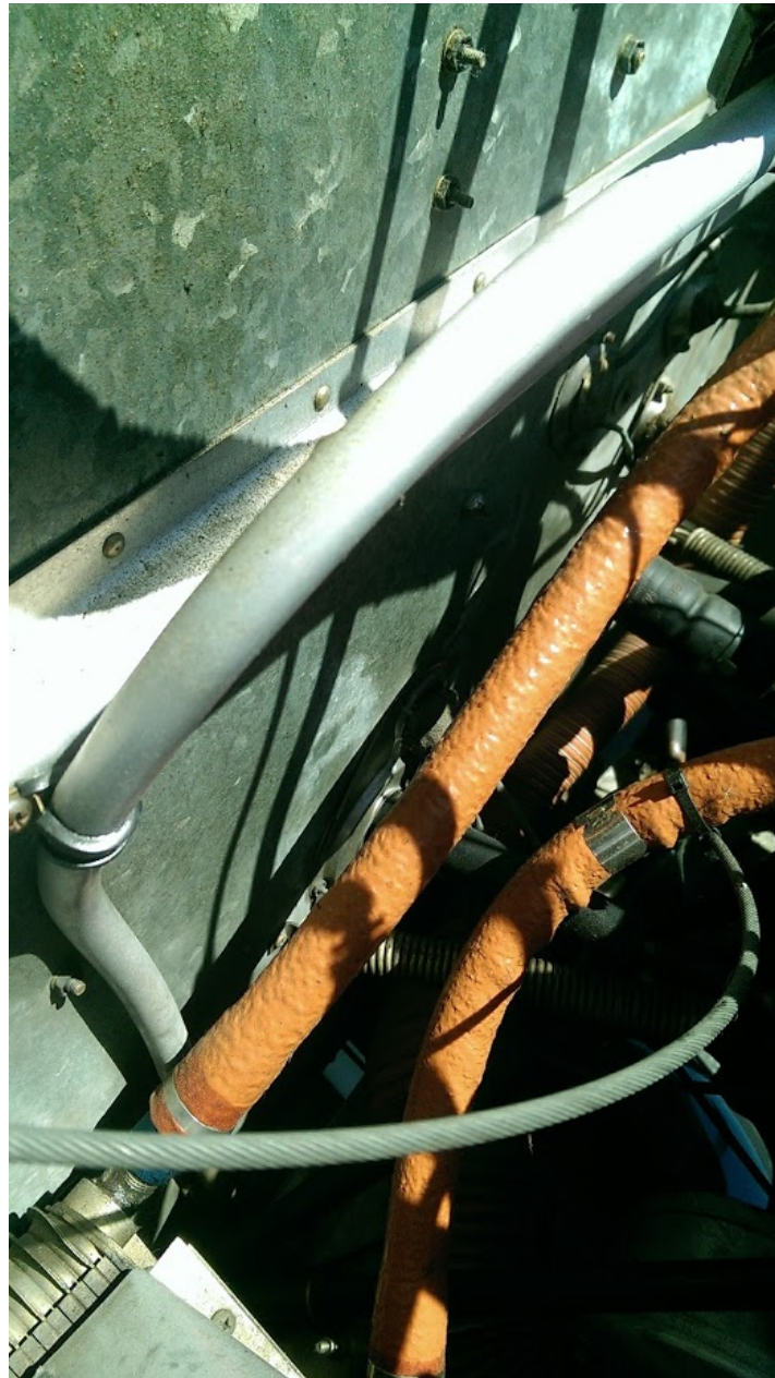
Photo 1 – View of damaged firewall (photo courtesy of the FAA)
