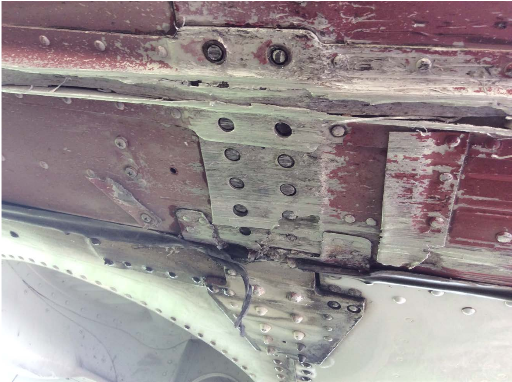
Photo 1 – View of damage to longerons (Courtesy of FAA)
