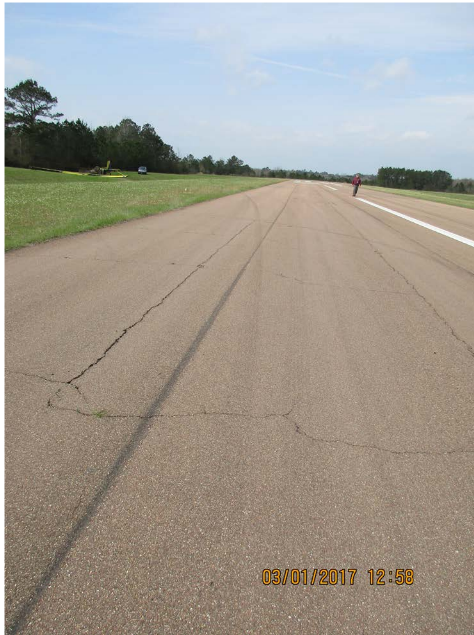
Photo 4 – Tire Marks Leading Off Runway into Grass (Photo Courtesy of FAA)
