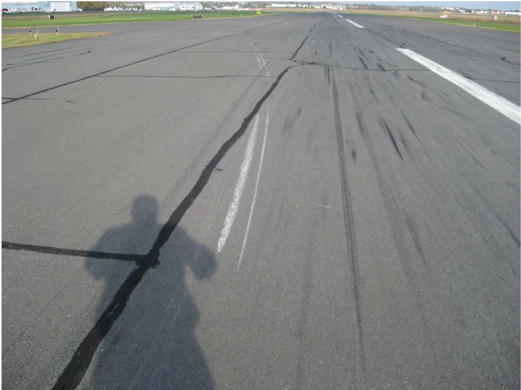
Photo 5 – View of white paint transfer on the asphalt of Runway 34 (Courtesy of FAA)
