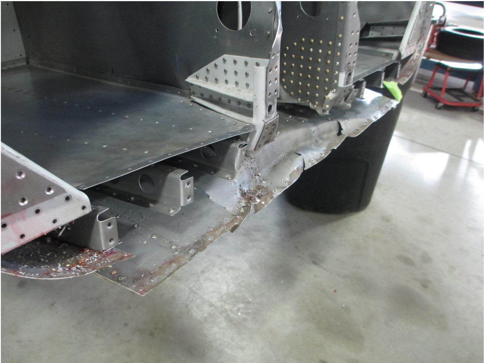
Photo 1 – Photo of damaged firewall bulkhead (Photo courtesy of the FAA)
