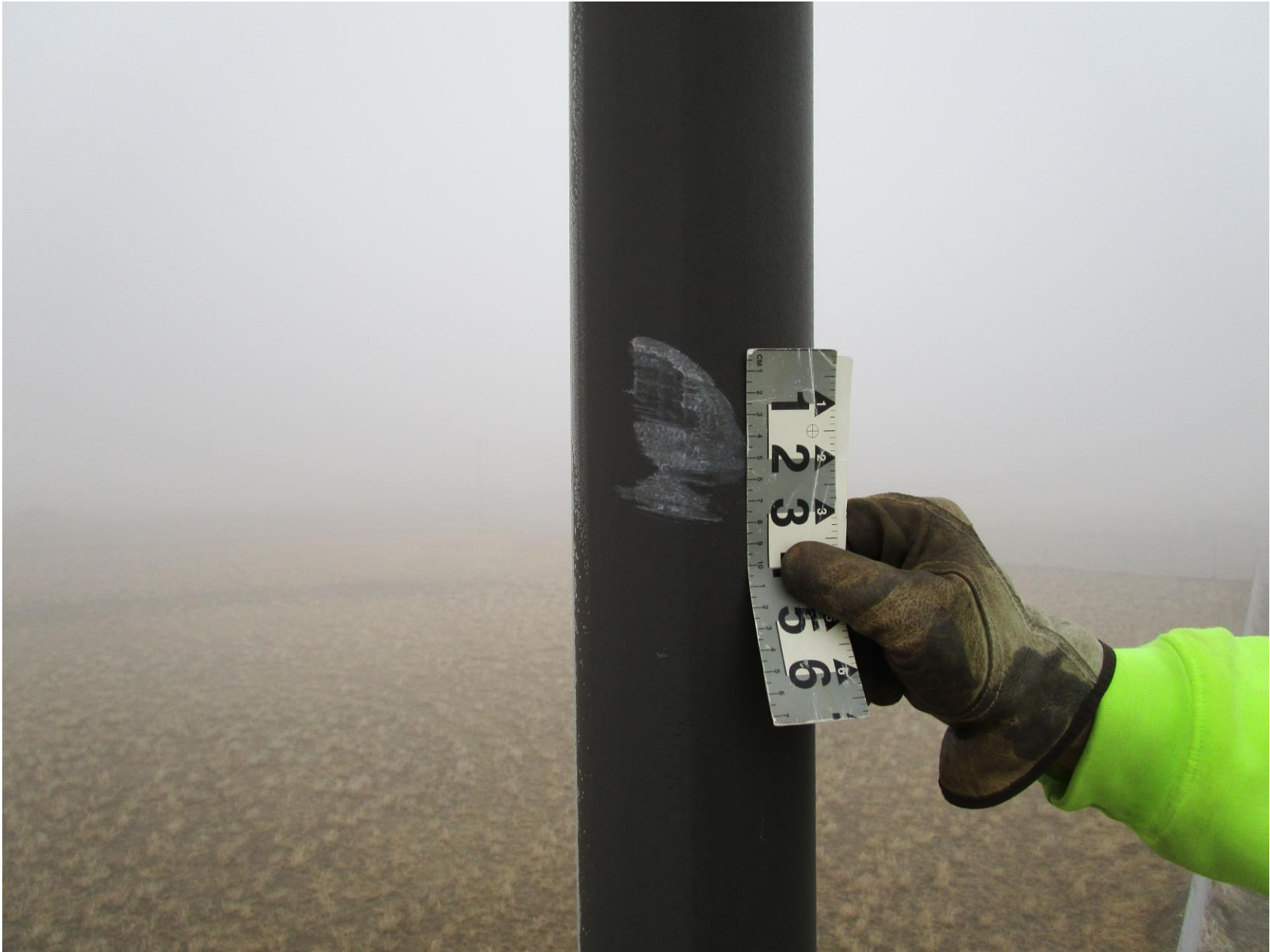
Photo 7 – View of light pole impact mark (courtesy of the FAA)
