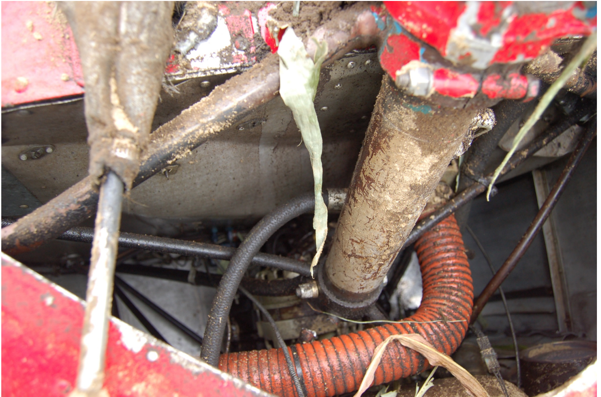
Photo 1 – Substantially Damaged Firewall (Photo Courtesy of FAA)
