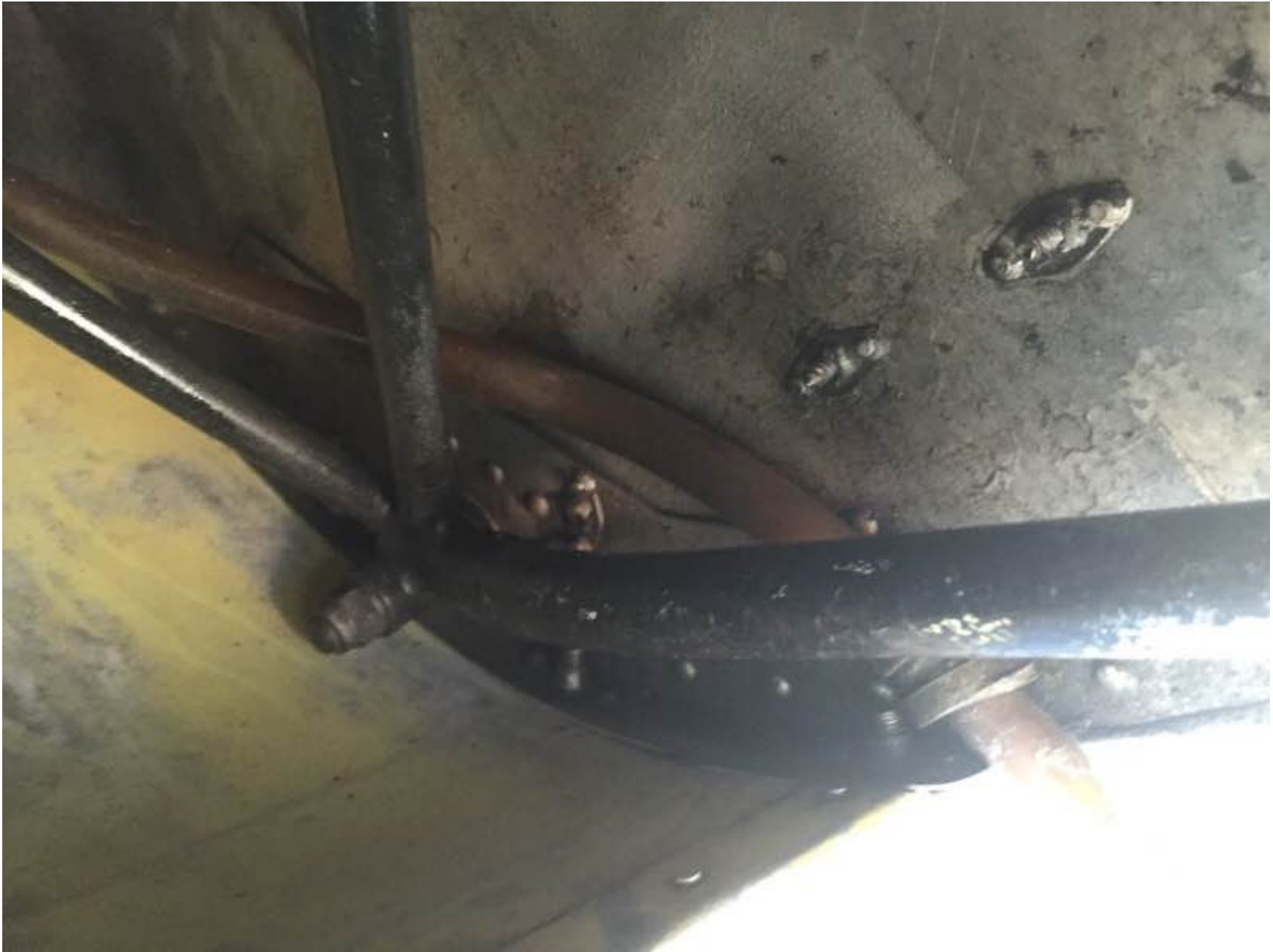
Photo 2 – Substantially Damaged Firewall (Photo Courtesy of Operator)
