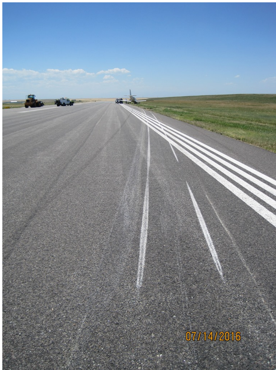
Photo 2 – View of white paint transfer on asphalt runway (Courtesy of FAA)
