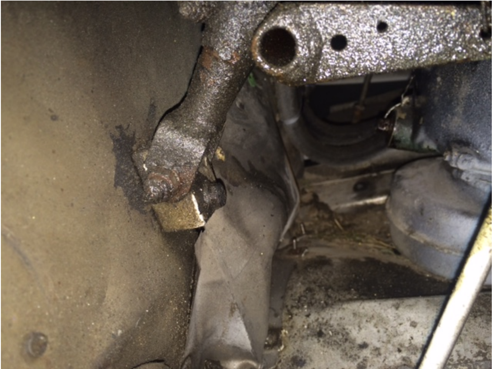
Photo 1 – Substantially Damaged Firewall (Photo Courtesy of FAA)
