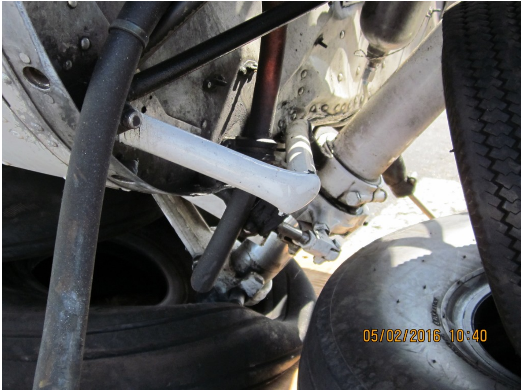
Photo 1 – View of damage to firewall (Courtesy of FAA)
