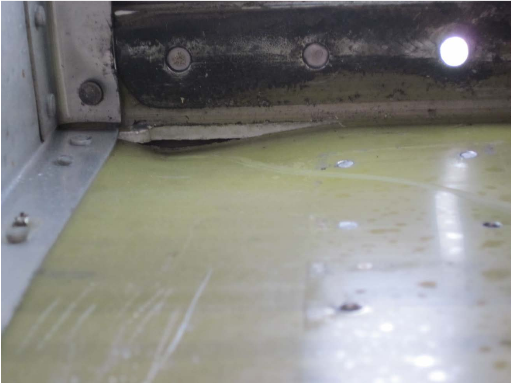
Photo 2 - View of damaged wing spar (photo courtesy of the FAA)
