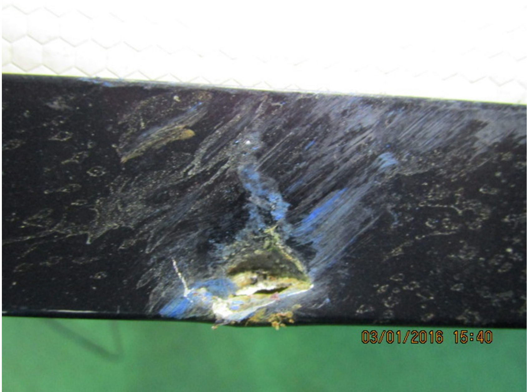
Photo 4 - View of paint transfer from Maule on to taxiway sign (Courtesy of Airport Manager)
