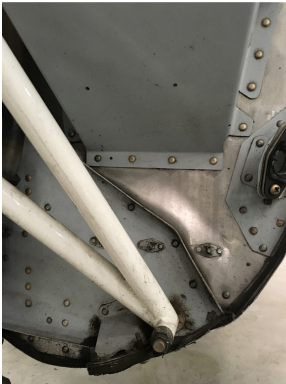
Photo 3 – View of damage to the firewall (Courtesy of FAA)
