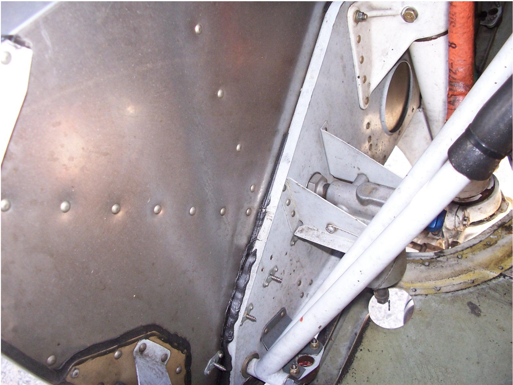
Photo 1 – View of firewall (photo courtesy of the operator)
