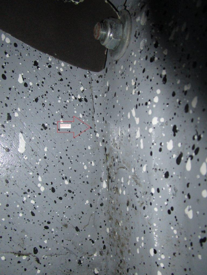
Photo 1 – Aft Side of Firewall Co-Pilot side (Courtesy of
