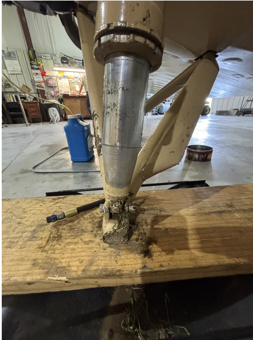
Photograph 4 - View of the left main landing gear. (Courtesy of FAA)
