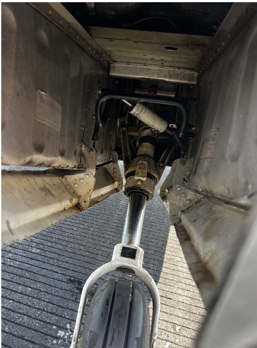
Photograph 2 - NLG tunnel damage (Courtesy of FAA)
