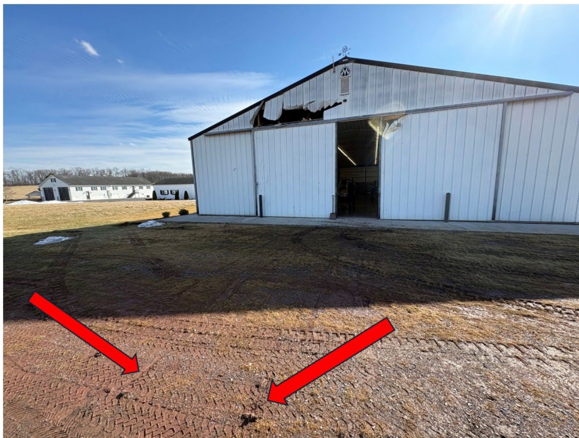
Photograph 3 - View of the Impacted Hangar and Area Where Helicopter was Located at Start of Liftoff. Arrows Point to Marks From Both Skids (Courtesy of Mr. Dickerson)
