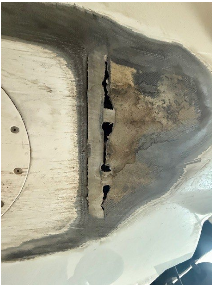
Photograph 2 - Lower Fuselage Damage (Courtesy of FAA)
