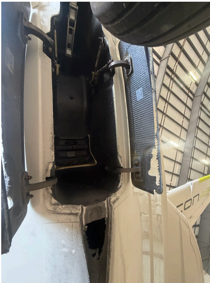
Photograph 2 - Damage to Nose Landing Gear Doors (Courtesy of FAA)
