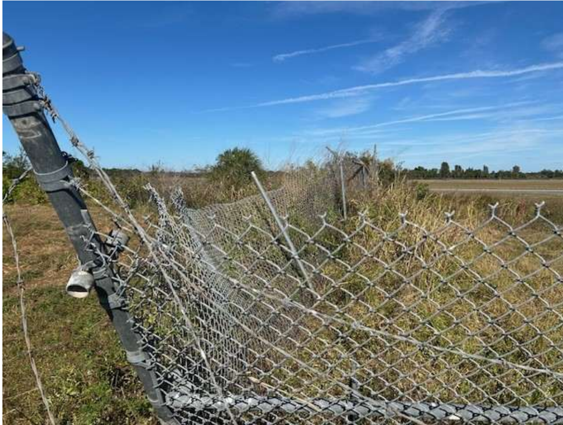
Photograph 3 - Section of perimeter fence impacted by the aircraft (Courtesy of Airport Authority)
