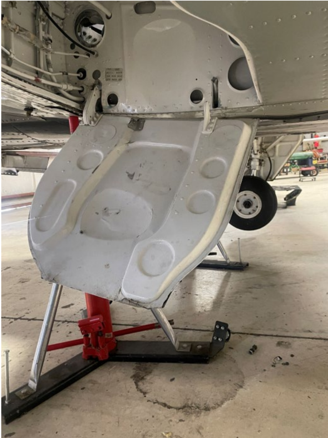
Figure 1: Left Inboard Main Gear Door
